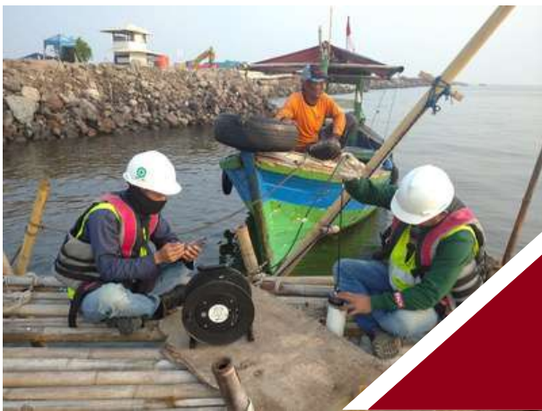
Monitoring Inclinator & Piezometer
